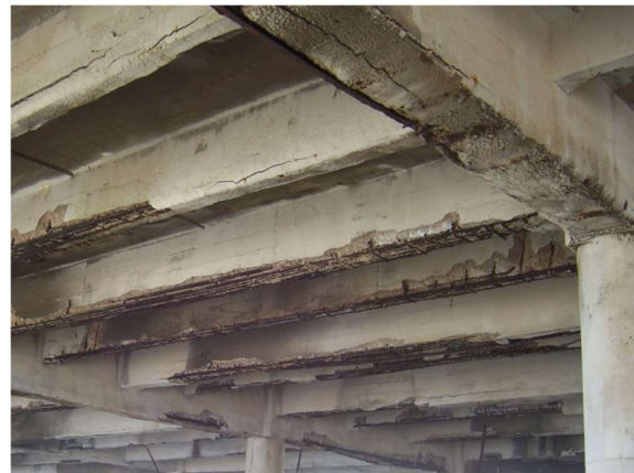
Figure 1 - Damage of concrete surface due to chloride and sulphate attack (Belkowitz J. , 2015).
