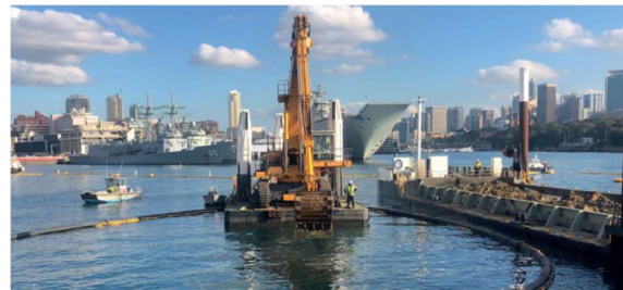
Figure 2 Birdon’s Backhoe Dredge loading contaminated dredging materials into Birdon’s split hopper barge at Garden Island (Source: [2]).
