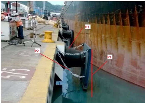
Figure 2 Three typical examples of poor fender system design
