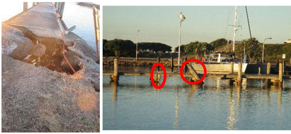
Figures 3a and 3b Damage at Crowdy Head harbour jetties due to seiche activity during the June 2016 storm
