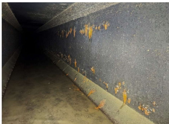
Figure 42 Tubercles concentrated in horizontal bands along the lower and upper parts of a tunnel wall. These represent areas with lapped reinforcing bars and have the highest steel density in the wall.
