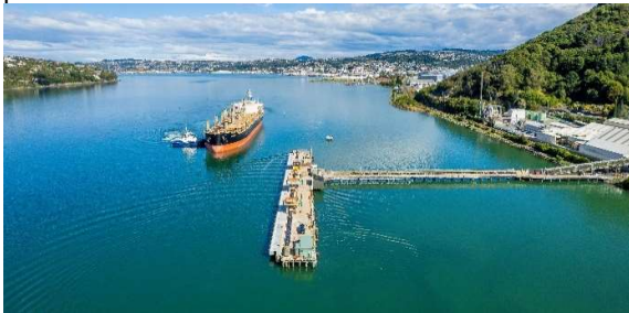
Fig 1 – Image of Ravensbourne Wharf and approach Jetty with vessel approaching newly strengthened structure
