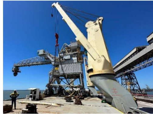
Figure 98 New Fully Assembled Shiploader Unloaded from Heavy Lift Vessel (HLV) and placed onto wharf rails in Gladstone, Queensland (Source: [3]).
