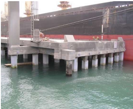
Figures 4 - shows the completed installation of pile jackets and repaired pile caps.
