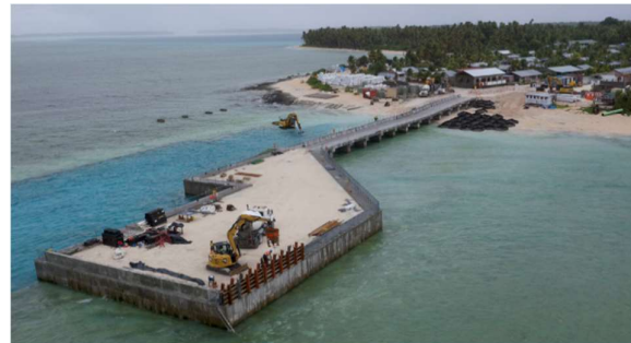
Figure 142 The blockwork structure of the wharf head and rock bag filled with dredged material next to accessway (Source: in house).
