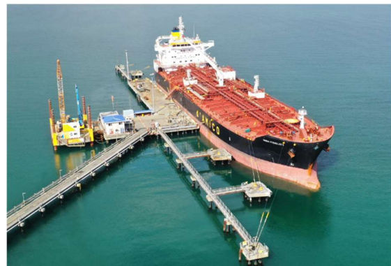
Figure 2 – Tanker berthed in Seaview while construction team is working on the barge.
