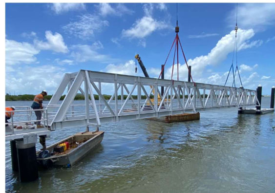
Figure 3: Dual 200t crane lift to install gangway from land only possible with the material choice being aluminium.
