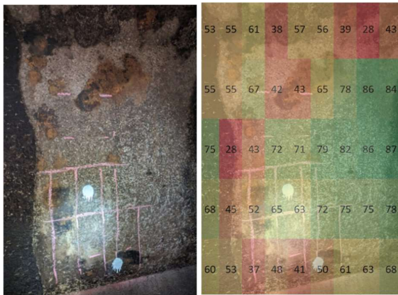
Figure 43 Tunnel wall shown (left) following pressure cleaning and (right) overlaid with concrete cover to reinforcement depth map (stated in mm) measured using GPR. There is a strong correlation between areas stained by tubercules and areas with lower concrete cover (identified as red/orange/yellow regions).
